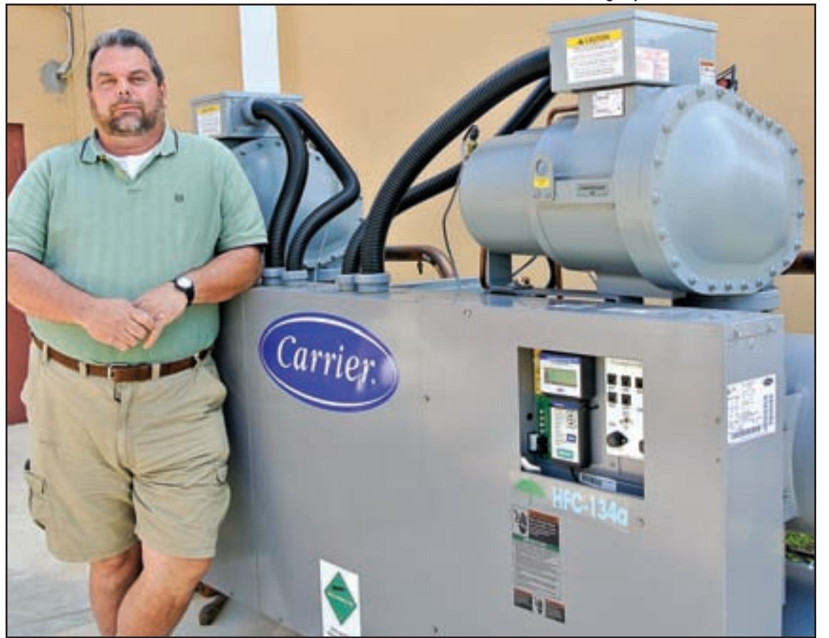
The new WPRF Club House manager poses with the new chiller.
