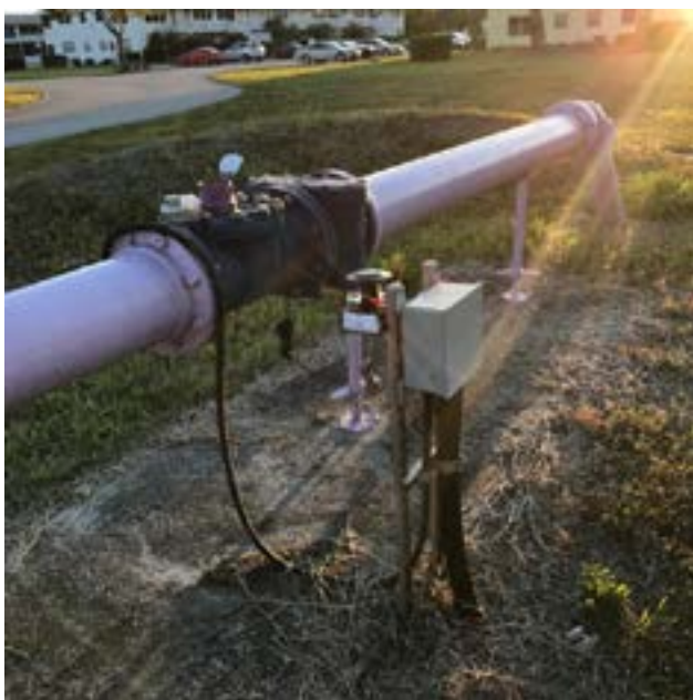
"THE LILAC PUMP"- THIS PUMP, AT NORTHWEST CORNER OF CENTURY VILLAGE, MOVES RECLAIMED IRRIGATION WATER INTO NORTH CANAL. ANY MECHANICAL COMPONENT OR PIPE THAT MOVES RECLAIMED WATER IS PAINTED LILAC PURPLE, TO ENSURE THAT THIS WATER IS NOT CONFUSED WITH POTABLE (DRINKING) WATER.
