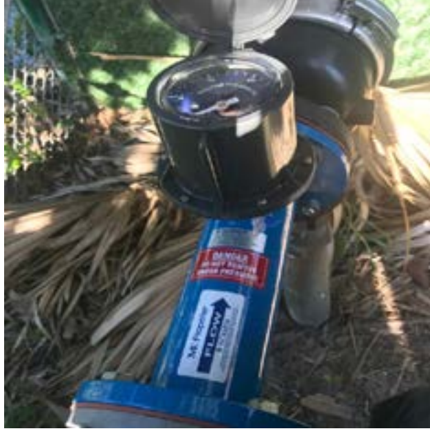
WATER PULLED FROM LAKE IS METERED- REPORT IS SENT TO SOUTH FLORIDA WATER MANAGEMENT DISTRICT EACH MONTH. THESE METERS MUST BE RECALIBRATED OR REPLACED EVERY FIVE YEARS.
