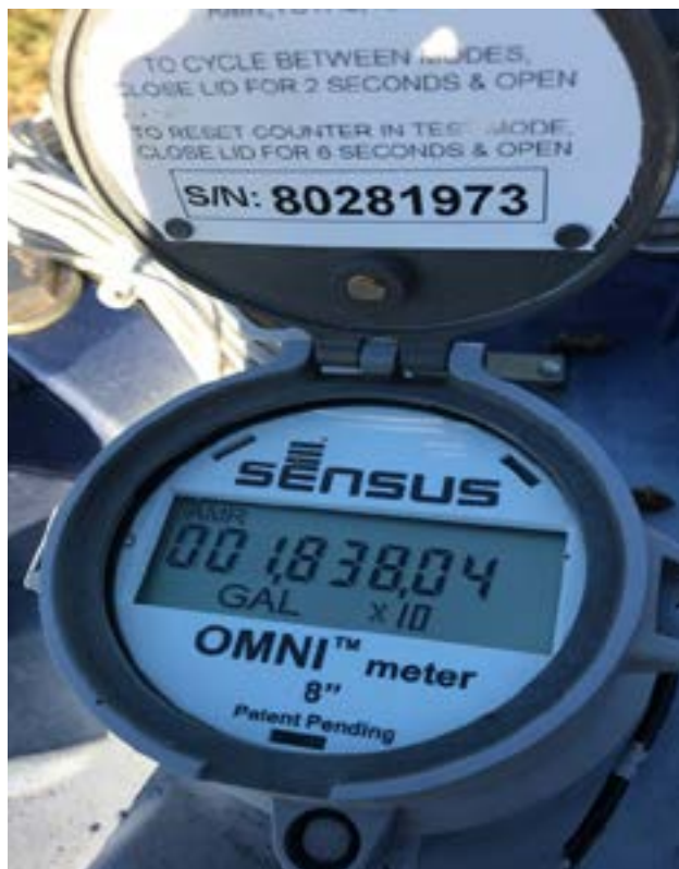
INCOMING RECLAIMED WATER IS METERED BY PALM BEACH COUNTY WATER UTILITIES. THE BILL IS SENT TO UCO.
