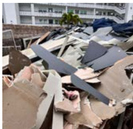
WELLINGTON K- THIS ASSOCIATION MADE SURE THAT THE UNIT OWNER'S CONTRACTOR BROUGHT HIS OWN DUMPSTER AND REMOVED THE DEMO DEBRIS.
