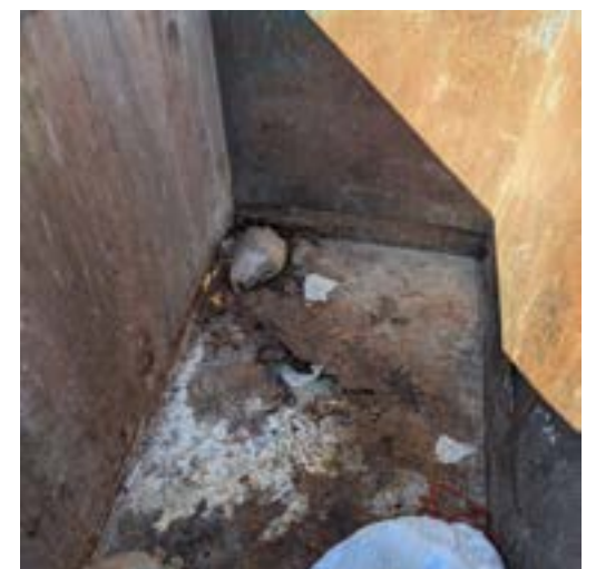
CAMDEN N- DUMPSTER WITH RUSTED OUT BOTTOM. A REQUEST FOR REPLACEMENT WAS SENT TO WASTE PRO. PLEASE SEND BUSTED DUMPSTER REPORTS TO UCOGARBAGE@GMAIL.COM. PICTURES ARE VERY HELPFUL.
